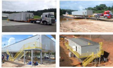
Figure 85 Modular electrical substation – transport and assembly
